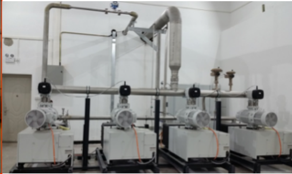
2K pumping system
